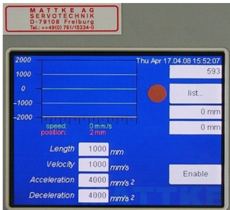
Touchscreen display on the control panel
